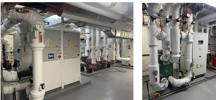
Figure 10: Chiller for Geo-Thermal System/Domestic Hot Water with CO2 heat pump as lead
